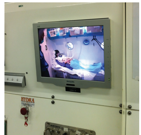
CCTV MONITORING SYSTEM
